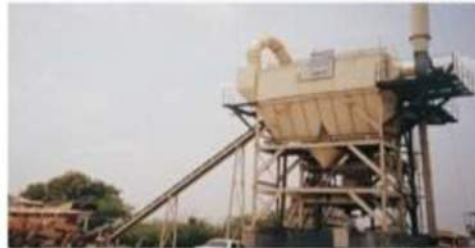
Hot Mix Plant
