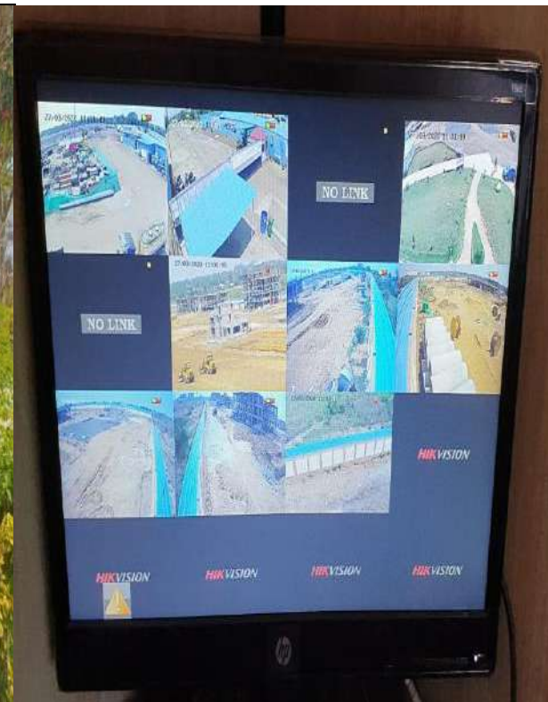
CCTV Monitoring for GMC Chandrapur
