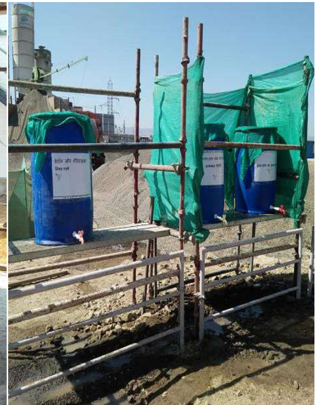
Common Hand Wash facilities at Joyville Hinjewadi
